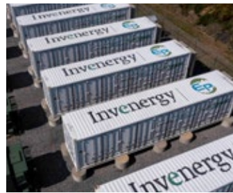
Storage: 21 projects; ~0.5 GW / ~1.8 GWh
